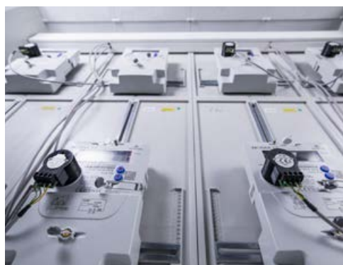
Meter box with installed optical couplers in the basement of the settlement on Hosemannstraße in Berlin Prenzlauer Berg
