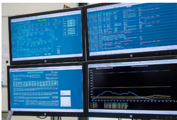
Screens in the grid control centre © ahnenenkel.com/Silke Reents
