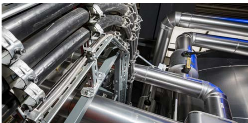
Beautiful co-existence: electricity and water lines at the energy hub. © ahnenenkel.com/Silke Reents
