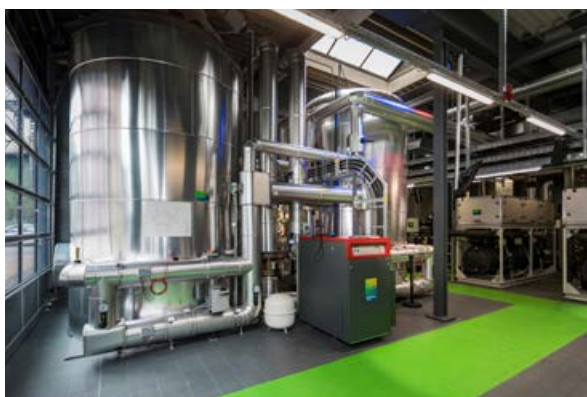
The heart of the energy hub with large reservoirs for hot and cold water. © ahnenenkel.com/Silke Reents
