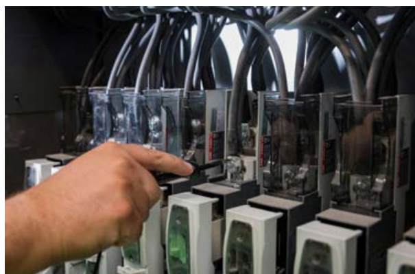
Individually protected: the power supplies for individual heating components in the large flow heater. © GASAG
