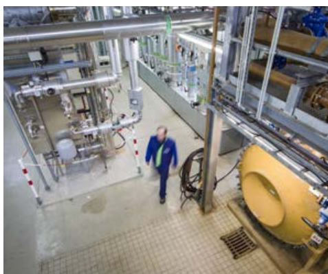
Technicians in the CHP hall
